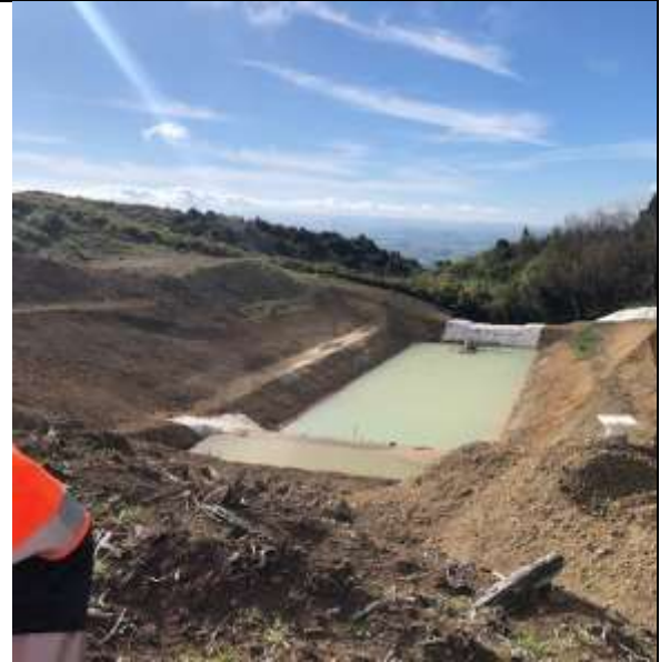
Figure 8. Chemically dosed sediment retention pond
