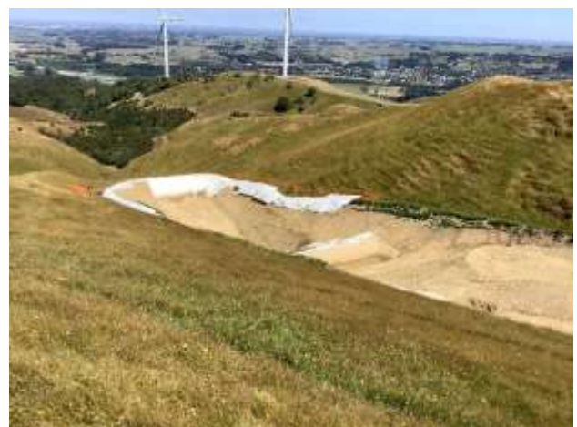
Figure 5. Sediment retention Pond in Construction Zone 2.
