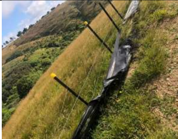
Figure 7. Impact of high winds on a silt fence.
